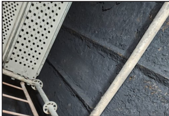
Corrosion inside bag house.
