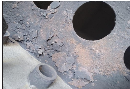
Severe corrosion at bag frame plate.
